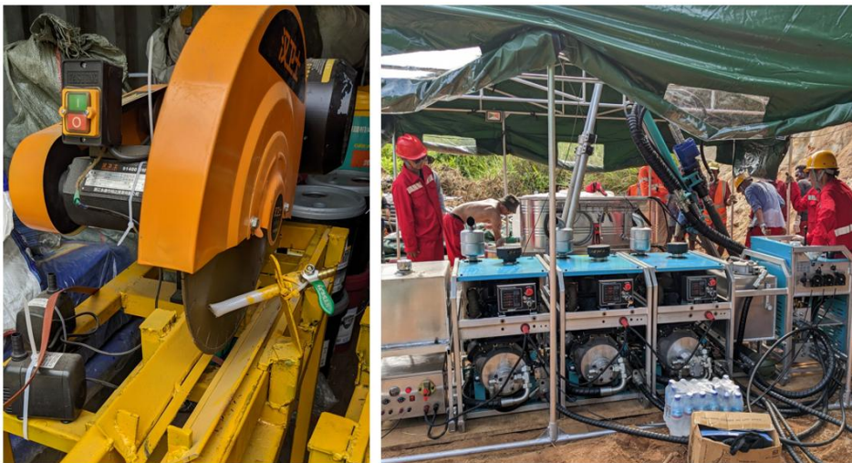
Figure 11-1. Core saw and drillrig set-up in December 2024 prior to commencement of drilling.
